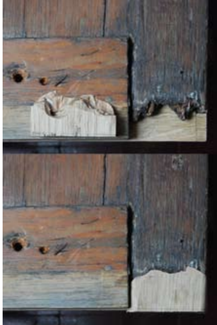
Figure 3. Loss compensation consisting of the fitted oak replacement and Araldite epoxy resin
